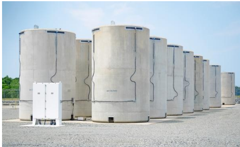
McGuire Station dry cask storage stores spent fuel on site
